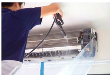
Air conditioners need regular servicing
